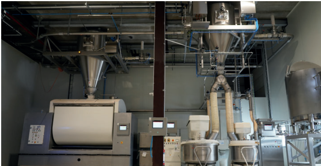
The dough chambers are equipped with a convenient dust extraction system, making for a much more pleasant work environment.
