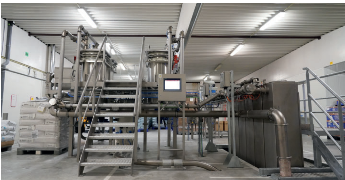
Climate-controlled tanks, transportation pipes, weighing and dosing equipment, and mixers are controlled by a fully configurable recipe management and production control system.
